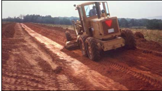
Soil excavated when forming the channel is used to construct the berm
