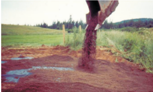
Figure 2. Gravel is added on top of geotextile without driving onto the material.
