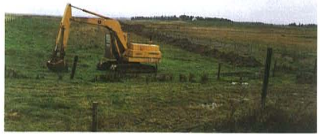
Figure 13. A Typical Excavator that was used to Construct the Open Ditch in the Right of the Figure.
