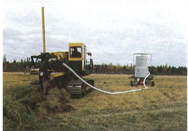
Figure 17. Laser Receiver Mast Mounted on a Trenchless Drainage Plow, 100 mm (4 in.). Filtered Tubing Being Installed.
