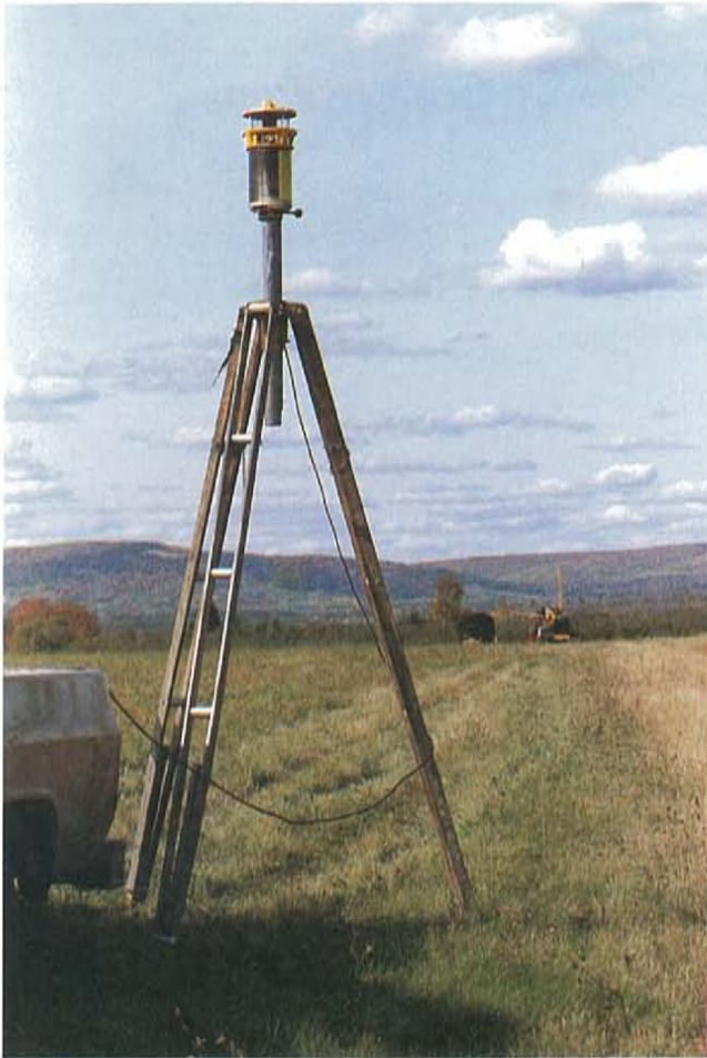
Figure 18. Laser Grade Control Emitter Tower. Note the Drainage Machine in the Background.
